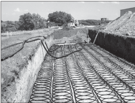
A horizontal loop field can be less expensive than vertical drilling, but requires more space, as shown at this electric co-op installation.
